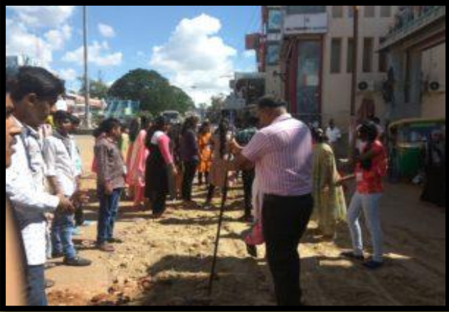
Department of NSS organized Shramadhan on 1 st October 2018, students covered the potholes on the roads with mud
