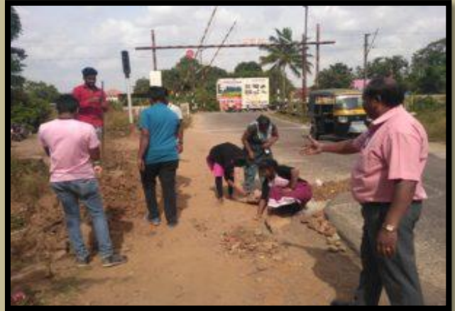
Shramadhan Programme was organised on 27 th July 2017, by NSS in Oorugum railway station road, students covered the potholes on the road with mud and made convenient for the people who travels
